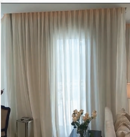
MOTORIZED WINDOW BLINDS CLIENT : PRIVATE CLIENT
